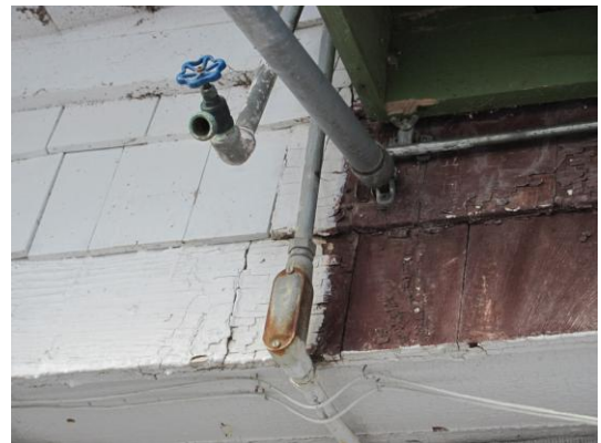
Without a define exterior aesthetic that is based on architectural history and understanding by maintenance staff of why and where certain paint colors should be applied, situations like this result where the historic stained shingles are partly coated with the universal “white paint.”
