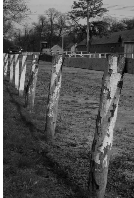
The original timber fence lining the historic Horse Haven track. Many timber members have been removed and replaced with 4" x 4" posts. The original timber design should be reconstructed.
